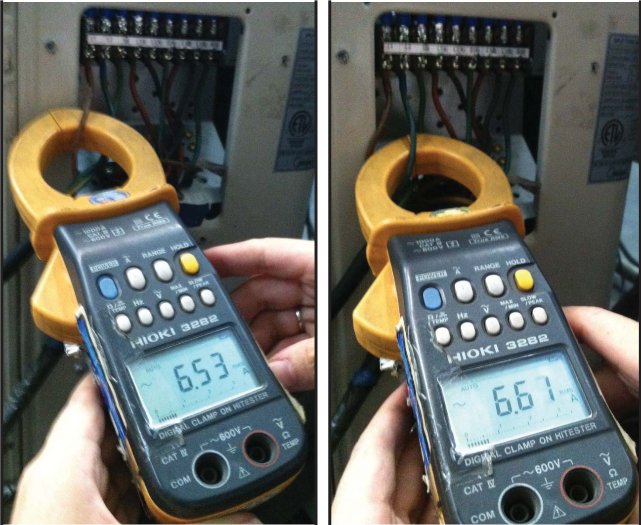
Fig. 61 – Test the voltage
