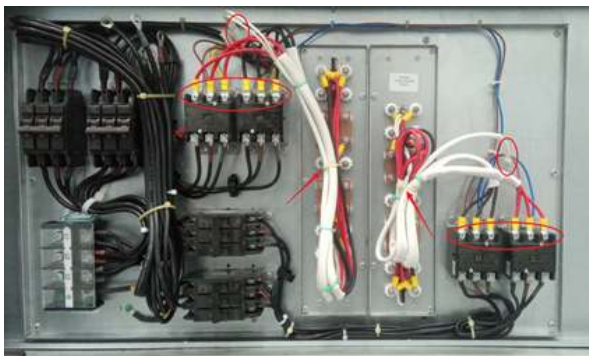
Figure 6. Electric heater wiring
